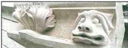
One of the replacement pieces of masonry soon to grace Lichfield Cathedral. (AK200210-0204A)
