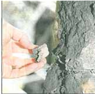
Cathedral architect Robert Kilgour points out areas of decay on one of the flying buttresses. (CS170409-3987LM)
